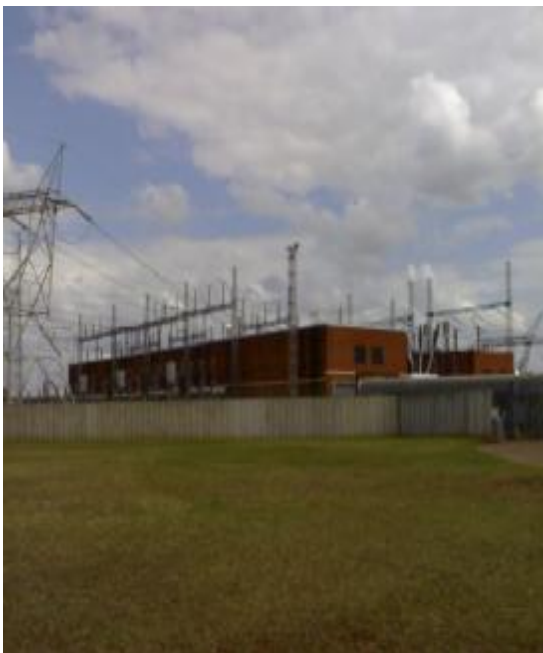
Photo 2: Photo of Invubu Substation
